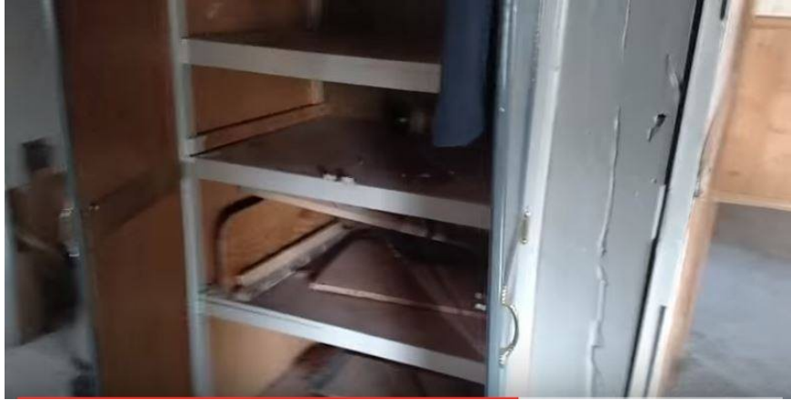
Stepping FORWARD into kitchen, turning RIGHT & looking into dirty cupboards.
