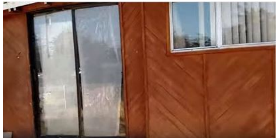
Closeup of front of house showing uncared for conditions.
