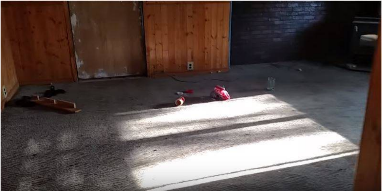
Facing OPPOSITE DIRECTION from previous photo, then stepping FORWARD into the living room; old food on the floor, thick dust.
