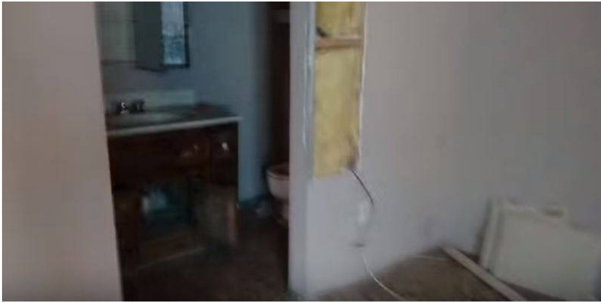
Stepping to the LEFT & looking UP from previous photo into the restroom, as discovered.
