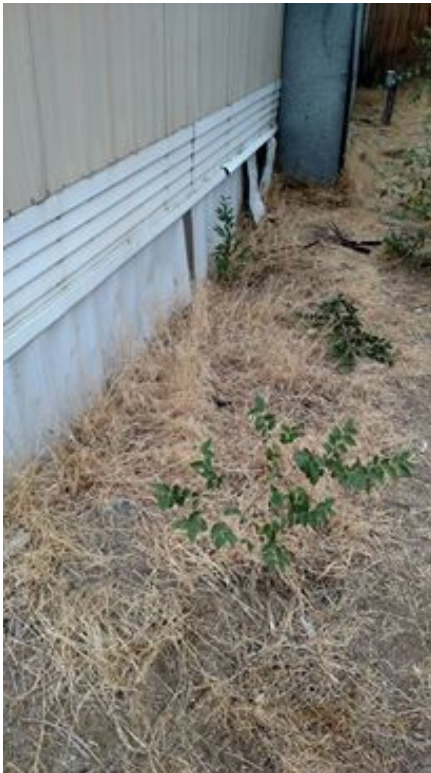
Invasive shrubs growing along west side of house, with root systems aiming directly toward waterlines beneath the house--see photos on pages 56 & 57 for evidence.
