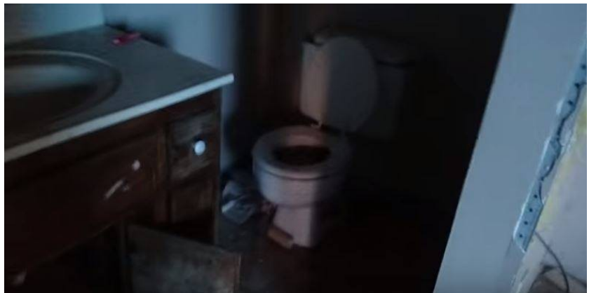
Stepping into restroom & looking DOWN & TO THE RIGHT from previous photo.
