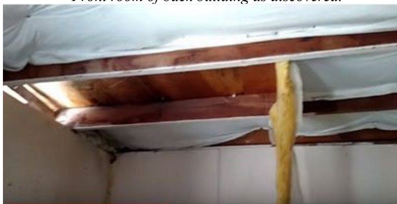
Insulation hanging from ceiling.
