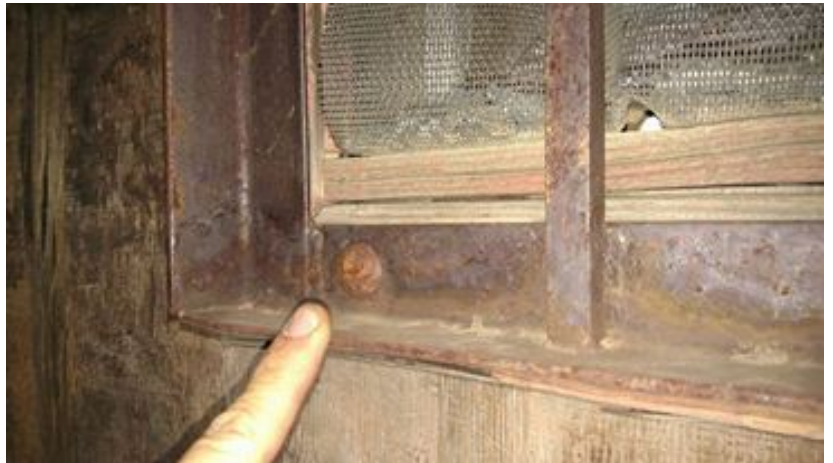
Closeup of LEFT barred window from above photo- glass window shattered.
