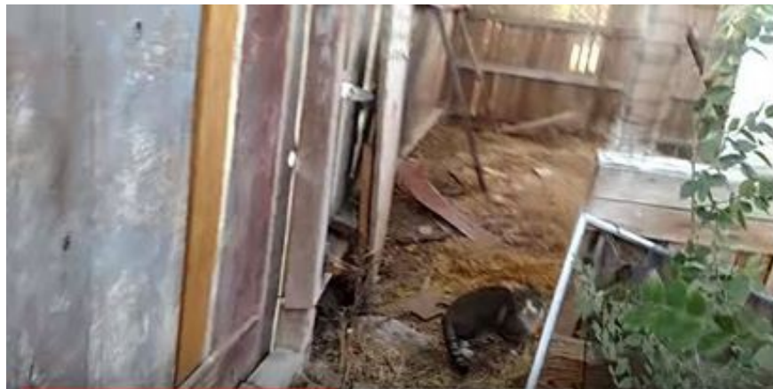
Stepping FORWARD from previous photo, showing debris on ground as found.
