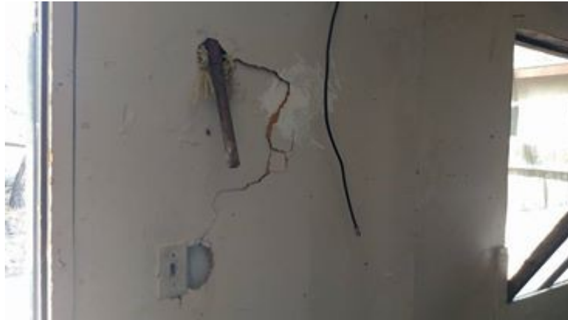
On LEFT SIDE of top photo on previous page, we see this wooden handle bashed into the wall as discovered.
