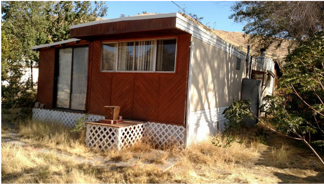
Dried grasses imposing fire hazard to main structure & wooden fences surrounding property, thus endangering neighboring properties.
