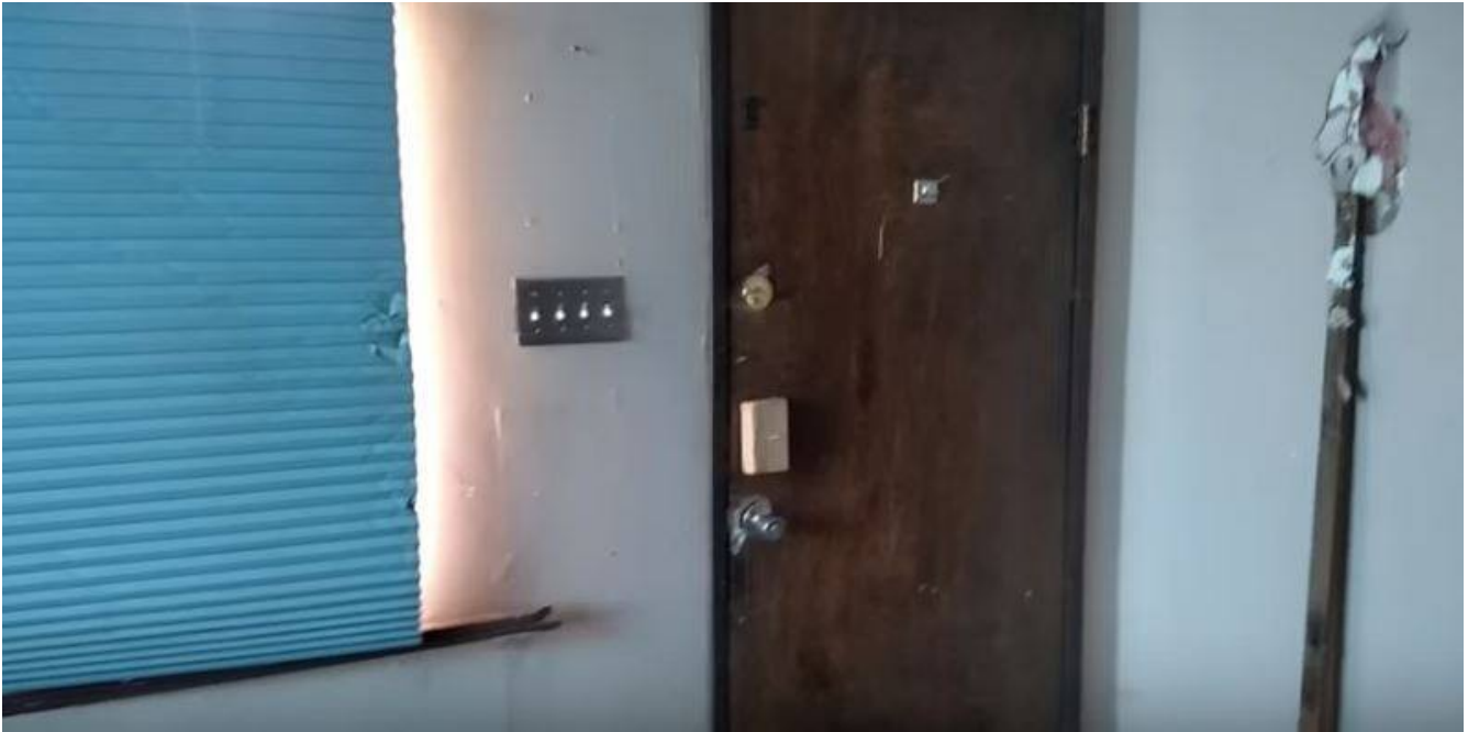
On the other side of the house from the previous photo in the back bedroom (through door in living room)- wall bashed in as discovered.
