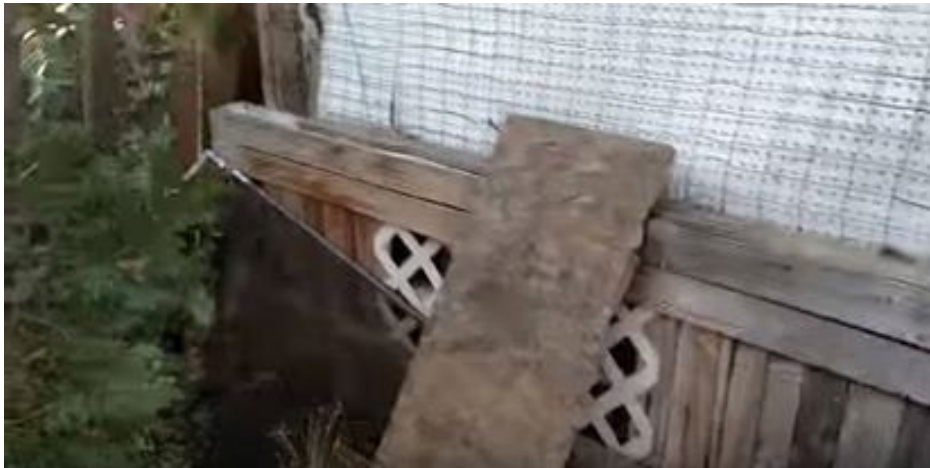
Looking to LEFT from previous photo- wooden contraption attached to house covered in debris.
